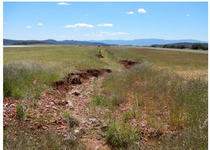
Example of Drainage Issues (Sedona Airport)
