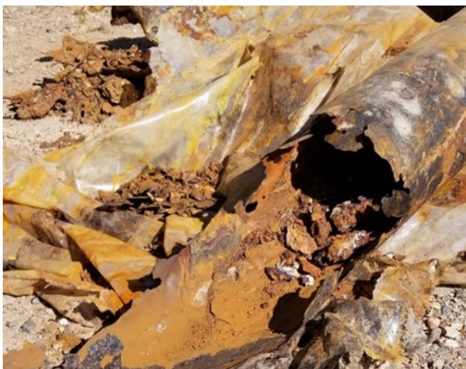
Section of Severely Corroded Pipe
