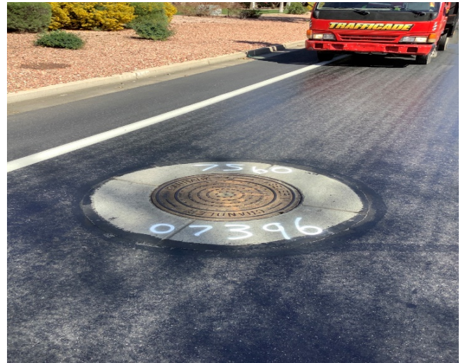
Standard View of Manhole within Right-of-Way
