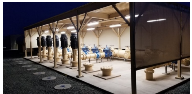
Booster Pump Station at Night
