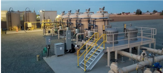
Nitrate Removal Facility
