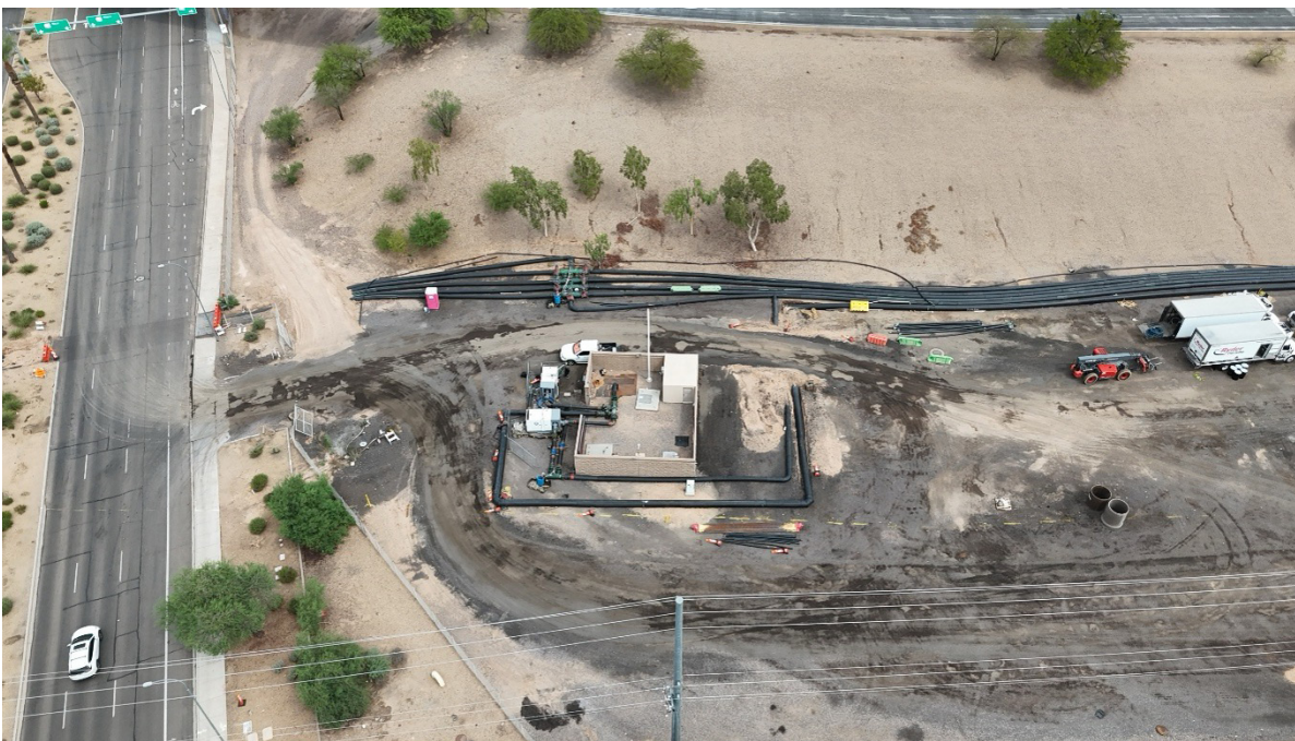
Figure 12 - Force Main Vault Bypass
